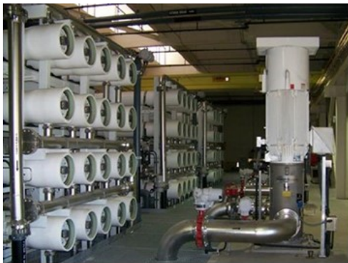
Banks of high-capacity reverse osmosis filters purify water for recharge into the aquifer.
